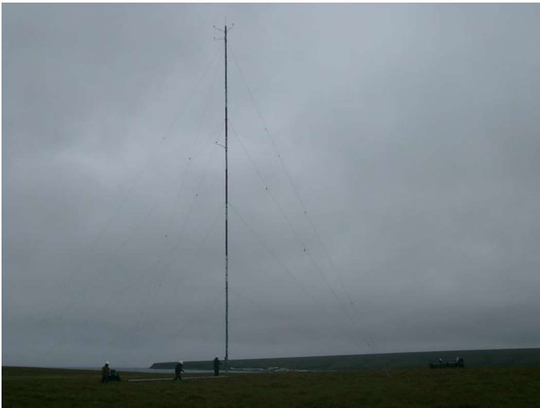
Installation of AEA met tower in Deering, August 2008 (photo by Brian Yanity)
