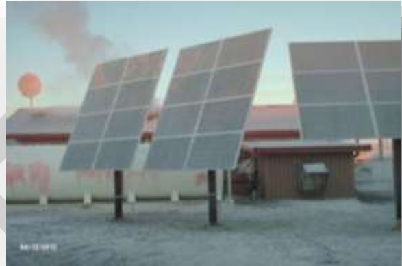
Ambler pilot solar project
