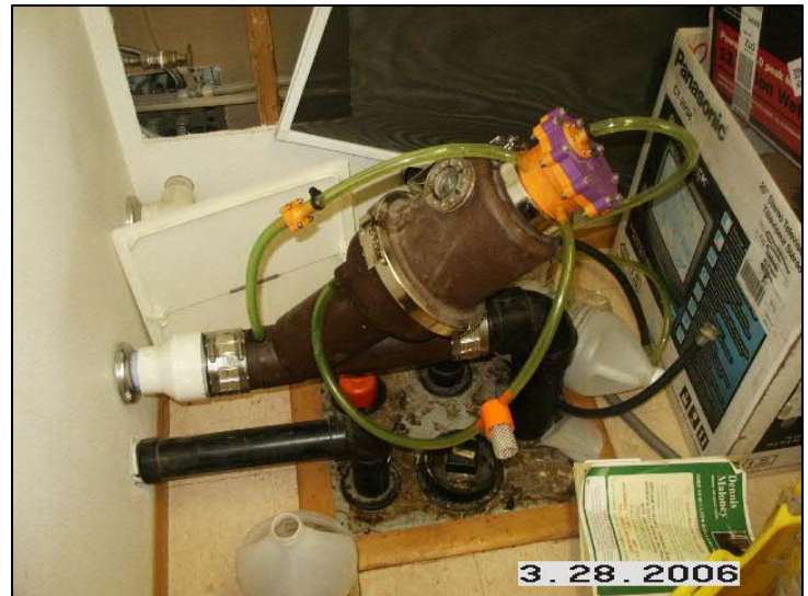
Figure 16: residential vacuum sewer unit.
